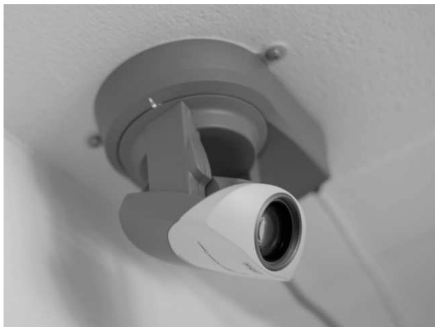
Figure 2: Pan/Tilt/Zoom camera mounted to the ceiling
